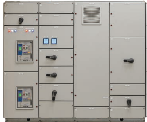
*Demonstration switchboard shown. Actual look and layout will depend on customer specification.
